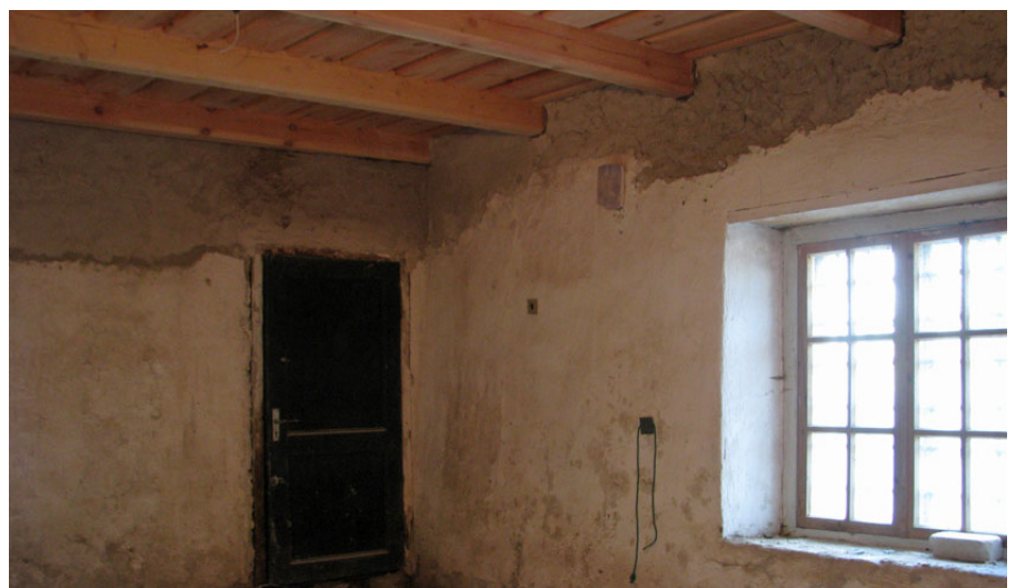
Much work is necessary in the interior
