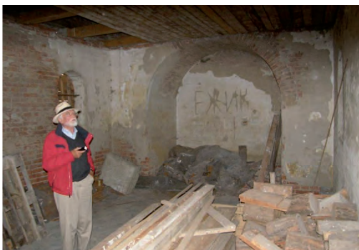
Miklós SvC viewing the damaged chapel
