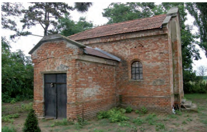
The chapel, provisionally repaired
