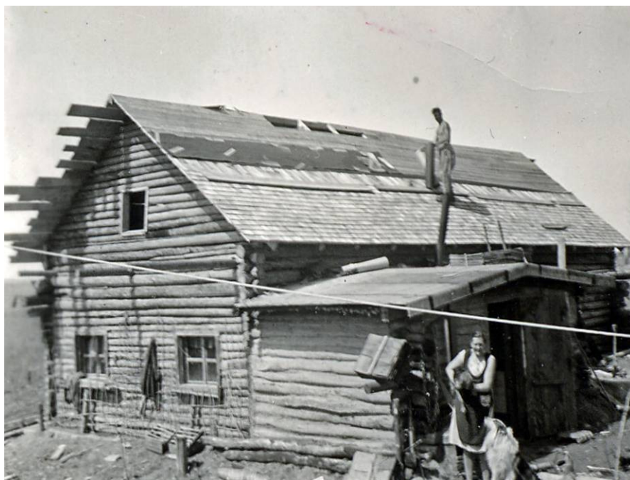
Gebhard von Schilling is roofing his cabin. At the bottom of the picture his wife Edith is working.
